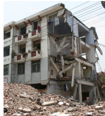
Fig. (9). A 4-storey building without sufficient tie beams collapsed at Dujiangyan.
