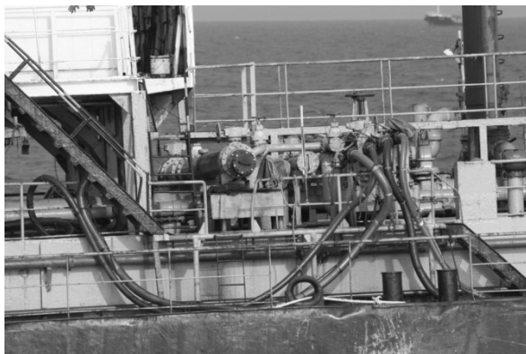
figure 7 equipment and oil pipe of oil tank
