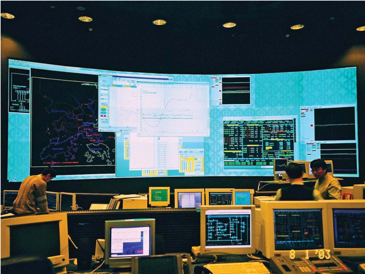
Figure 4-6 The System Control Center of CLP Power
