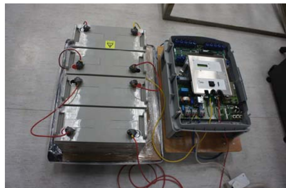
Figure 4-4 Smart meters for battery management
