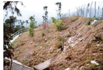
Planting failures, Shek O Road
