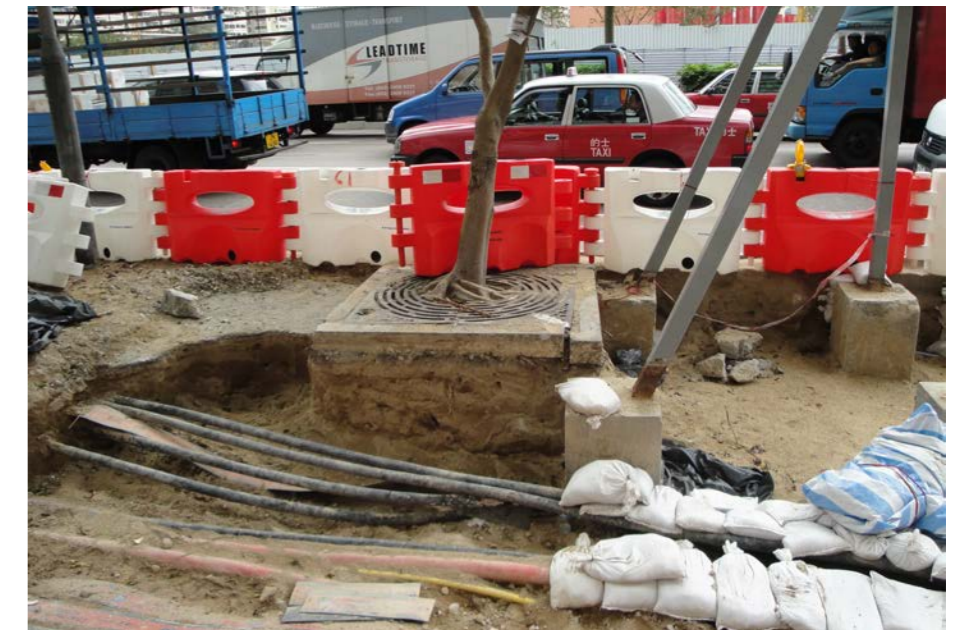
Extensive roadworks often threaten the roots and health of a tree
