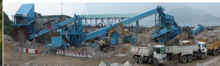
Tseung Kwan O Construction Waste Sorting Facility
