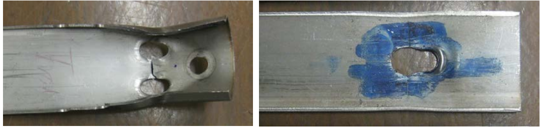
(a) Bearing and net section tension failure (A-S-3-8) (b) Bearing failure (T-D-1-12)
