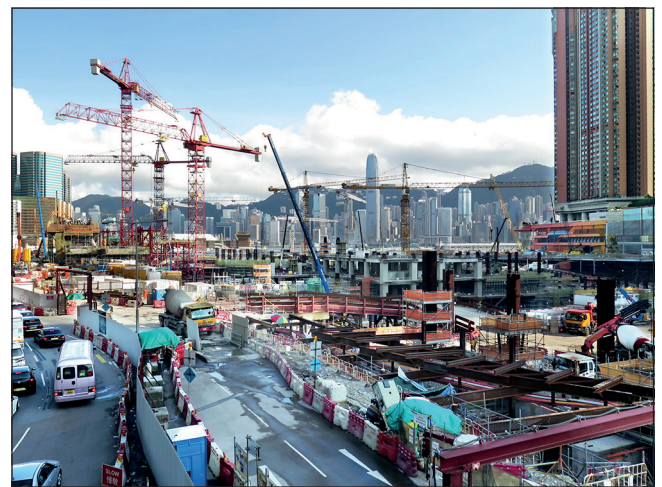
Figure 4. Construction site of West Kowloon terminus of the Guangzhou–Shenzhen–Hong Kong express rail link, which is due for completion in 2018 (By Wing1990hk (own work) (CC BY 3.0 ( http://creativecommons.org/licenses/by/3.0 )), via Wikimedia Commons)
