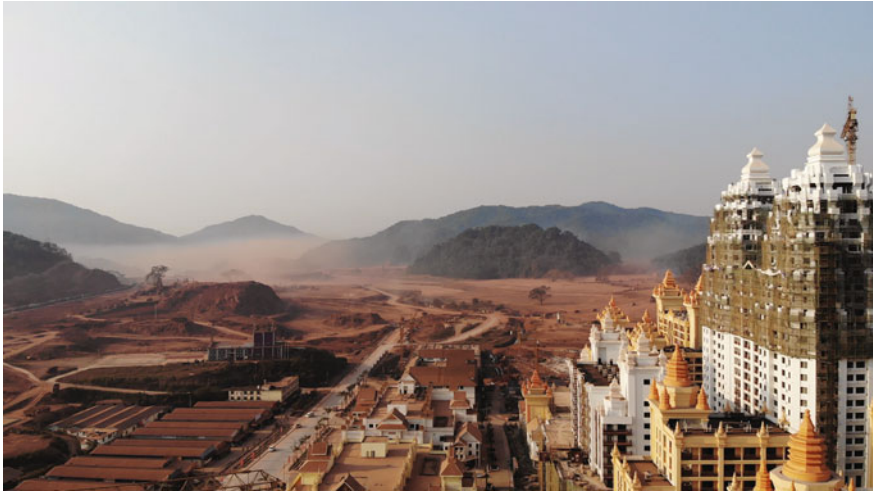
Fig. 2 Speed of construction within the Boten Special Economic Zone has accelerated since the inauguration of the Lao section of the Yunnan-Singapore railway, commonly called the China-Laos Railway. This photograph captured the ongoing construction and large-scale leveling of the landscape throughout the zone. Photo by Xiaoxuan Lu (March, 2019)
