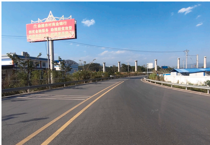
Fig. 5. Concrete viaduct columns under construction for the China–Laos Railway as seen from the Xiaomo Highway near Mansan Village in the Nanla River valley. Photo by the author.
