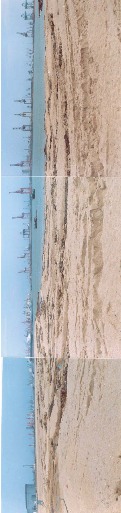
Fig. 6. Site photograph showing the slipped reclaimed land.
