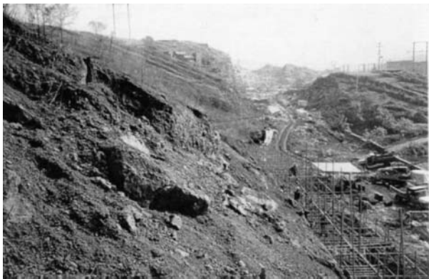
Fig. 2. Site photograph illustrating the general hilly terrain where the Yuqian National Expressway was being constructed.
