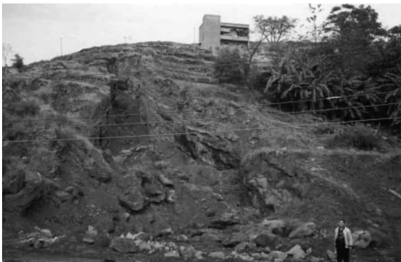
Fig. 4. The open gap and vertical and undulating tension cracks associated with the plane slide during construction of a national expressway in southeastern China, looking east. The open gap measured 6 to 8 m high, by 2 to 7 m wide and 53 m long in weathered mudstone overlying sandstone.
