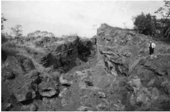
Fig. 6. A close view of the open gap and vertical and undulating tension cracks in the weathering mudstone with monoclinical beddings, looking east. Seepage from the bedding planes of the weathered mudstone is visible.
