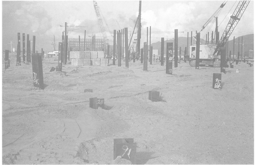
Plate 5. Sand fill, Type C, with steel driven H Piles for Cargo Terminal II. Type C was extensively used as a capping layer above -2 mPD in the reclamation of this part of the Southern Facilities Area
