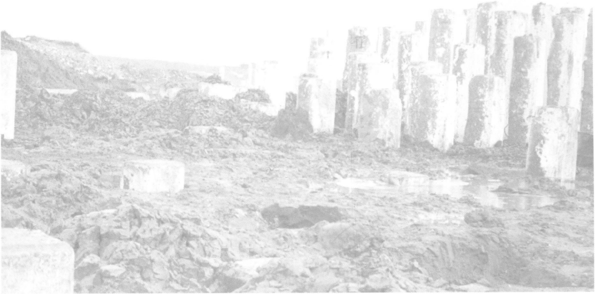
Fig.17. Some of the 20 000 piles driven to support the second phase of Drax Power Station in Yorkshire, UK
