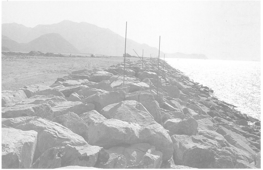
Plate 4. Hard durable Type A rock fill used as armourstone for the seawalls
