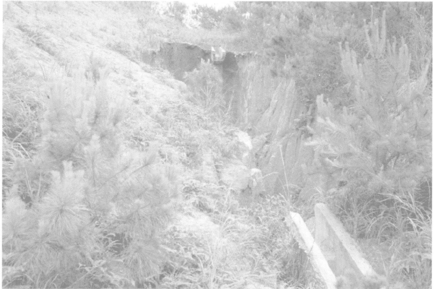
Fig. 5. Gulleying caused by slaking of completely decomposed rock (grade V)
