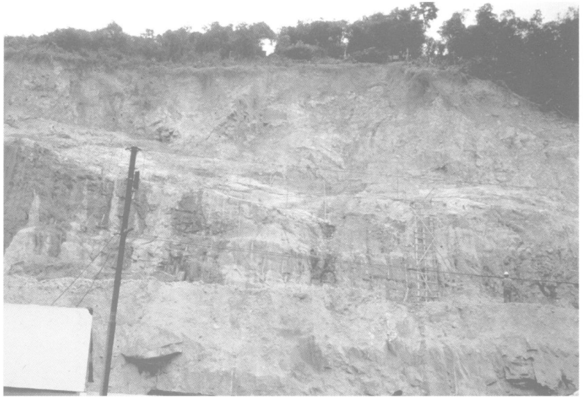
Fig. 14. Major rock slope failure at Repulse Bay, Hong Kong that occurred due to sliding within a zone of fractured rock and pink clay
