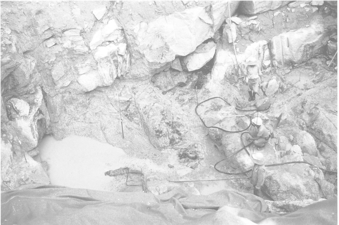
Plate 6. Cleaning of excavation for a pad foundation. Note variation in weathering and discontinuity pattern to be taken into account in RMR rating
