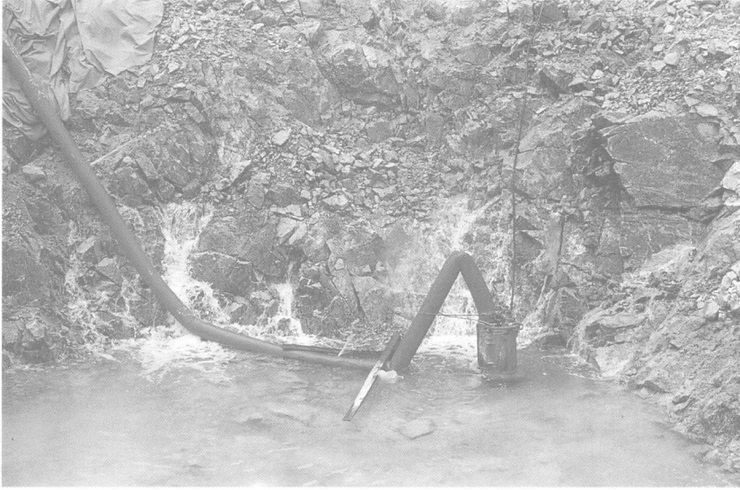
Plate 8. Excavation for road cutting through original Chek Lap Kok island. Note high groundwater inflow from high permeability zone created by fragmentation blasting
