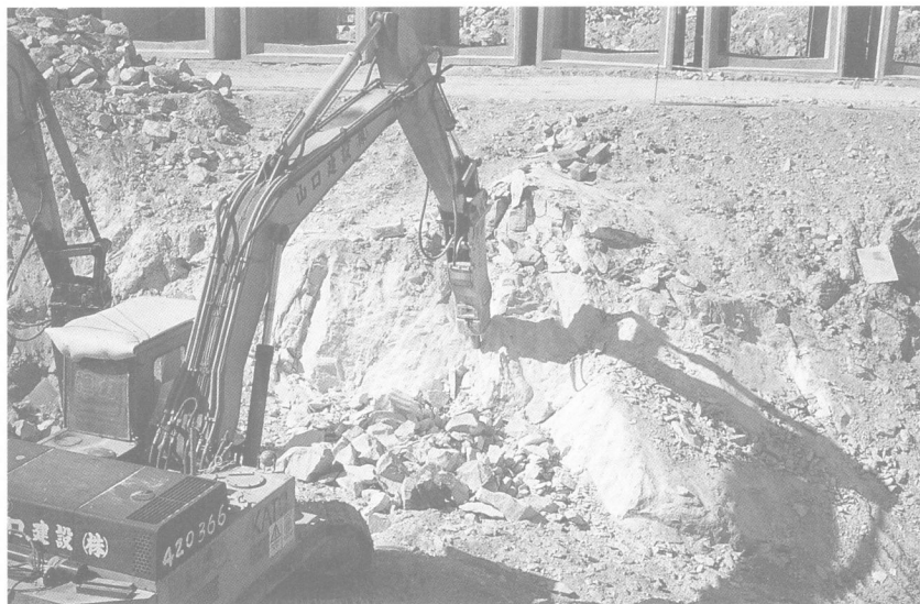
Plate 3. Trench excavation on original Chek Lap Kok island. Note rock exposure unbroken by fragmentation blasting, requiring subsequent break-up
